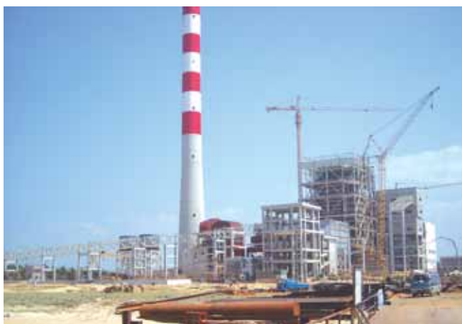
Puttalam Coal Power Station
