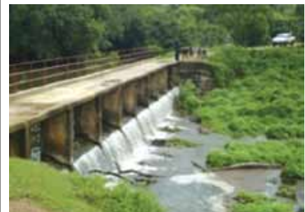
Mamaduwa Irrigation Scheme
